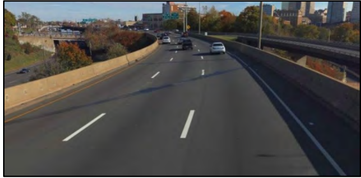
Deficient Left and Right Shoulders along I-84
