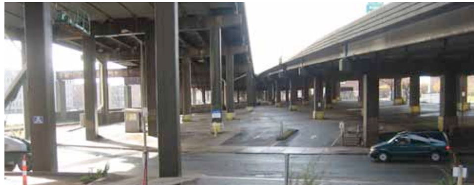
The Viaduct structure is nearing the end of its useful life and will need to be replaced.
